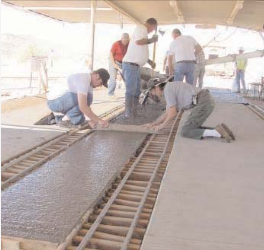
The Concrete Gang puts the finishing touches on the final pour in Adobe City Station.
